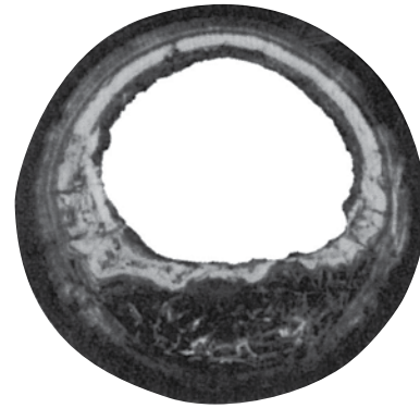
1/2 inch scale in 6 inch pipe, 1000 feet long, has a transfer capacity loss of 150 gallons per minute.
